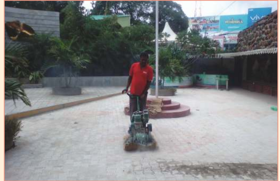
Ticket counter Interlock
