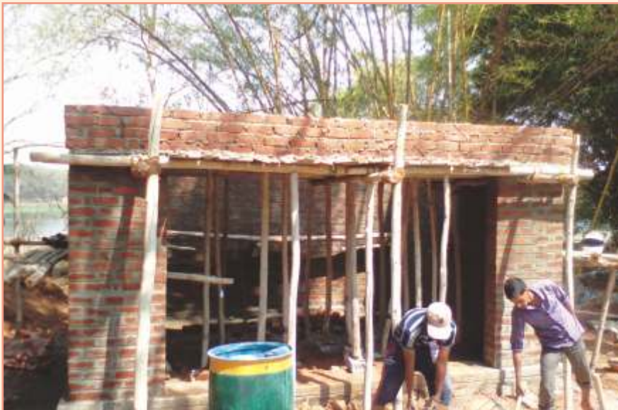
RO plant installation near karanji Boating Point
