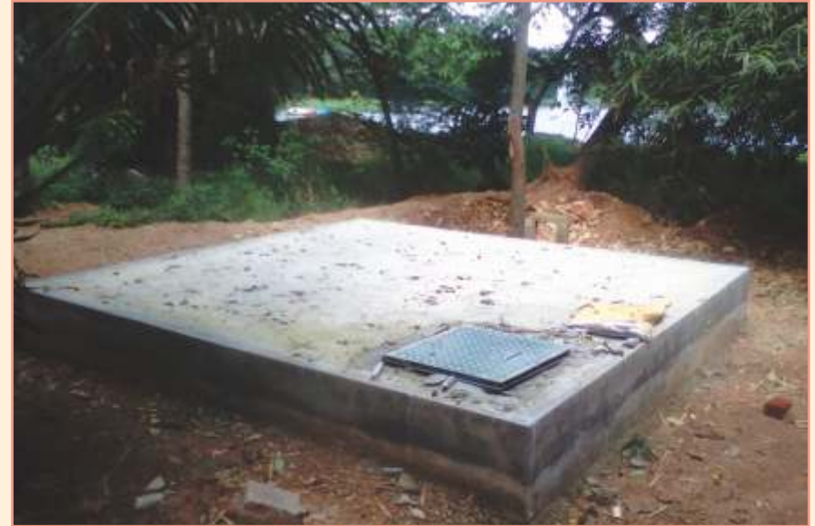
RO plant installation near karanji Boating Point
